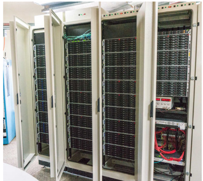
Figure 4. Rack front pic.
